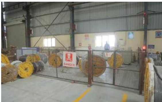
High Voltage Testing Area
