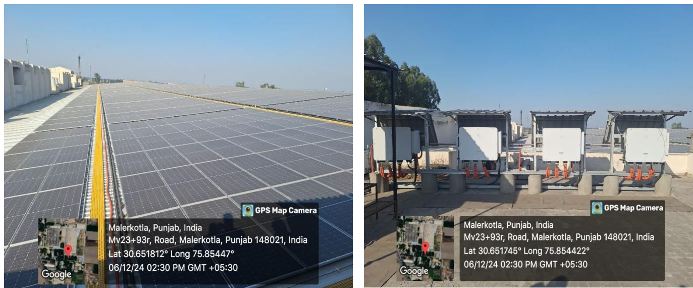
Existing solar plant of the company
